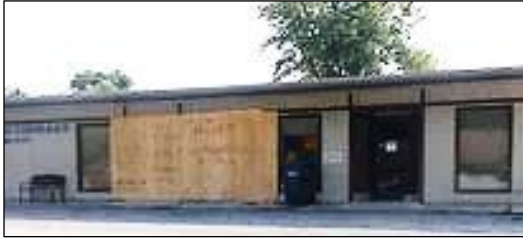
External damage to Library caused by 2014 truck accident. (Library photo)
