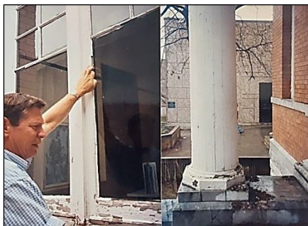
The Carnegie Library has required its share of repair and maintenance since 1905. (Library photo)
