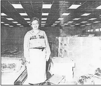
The new Library neared completion in the fall of 1997. Bethia Owens stands in the midst of the interior construction debris. (Sequoyah County Times)
